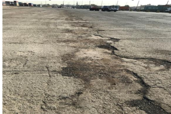
Figure 2: Transverse and long cracking
