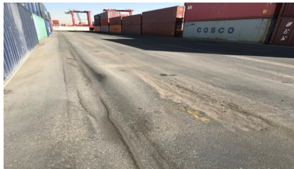
Figure 3: Pavement failure in containers yard
